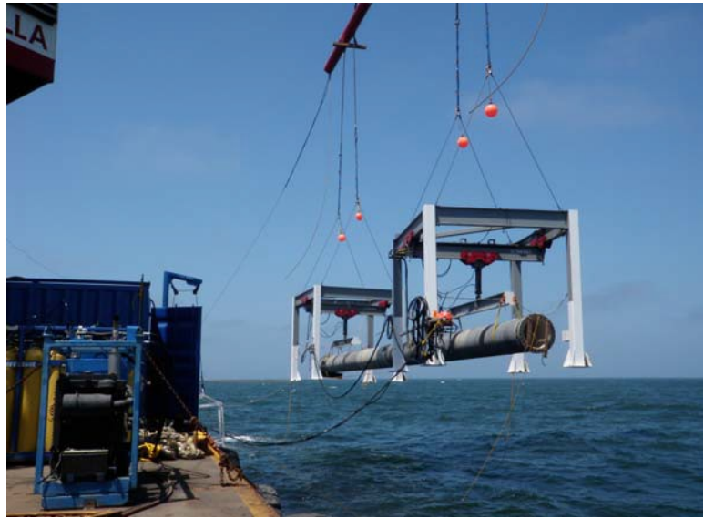
80' Spool Piece and Hydraulic "Horses" being lowered to be installed by HOI divers.
